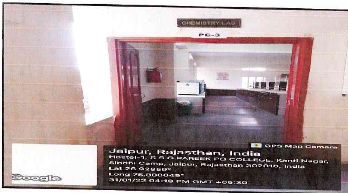
OUTER PHOTOGRAPH OF CHEMISTRY LAB-II
